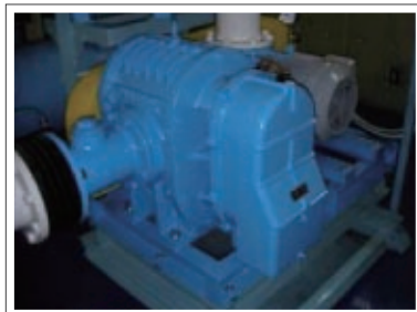
An inverter-fitted Roots blower newly installed in the toner production line
