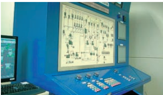
Operation state supervisory panel
