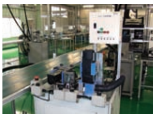
Inside view of a recycling plant
