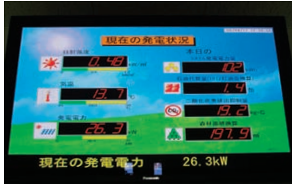
Panel indicating the level of power generation at this moment
