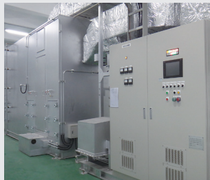
Waste gas treatment system
