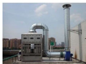
Newly Installed VOC Water Treatment System
