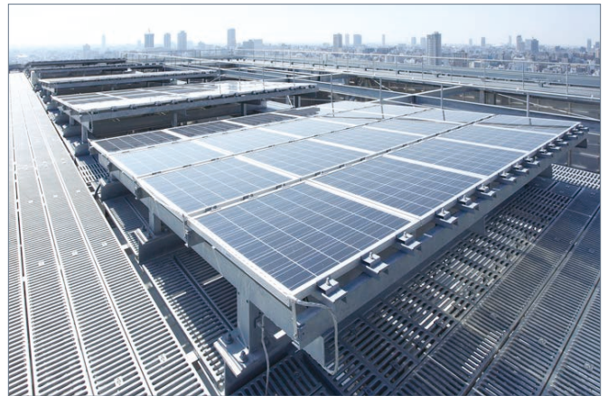
Solar electric generating equipment installed on the roof of the headquarters building (generated 13,614 kWh during 2012)
