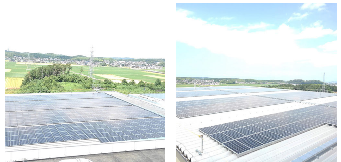
Solar power generation system on the plant building
